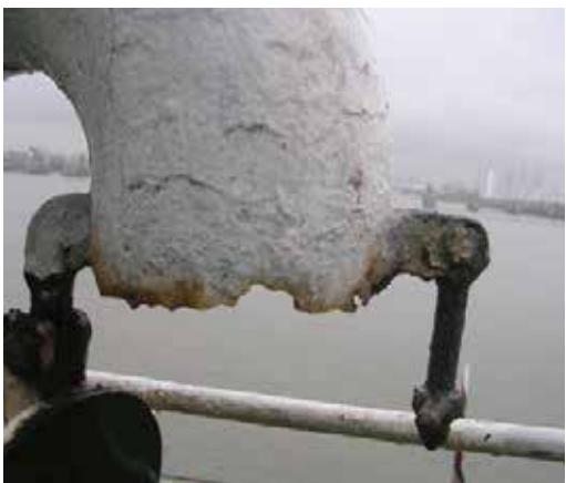
Wasted gooseneck air vent.
